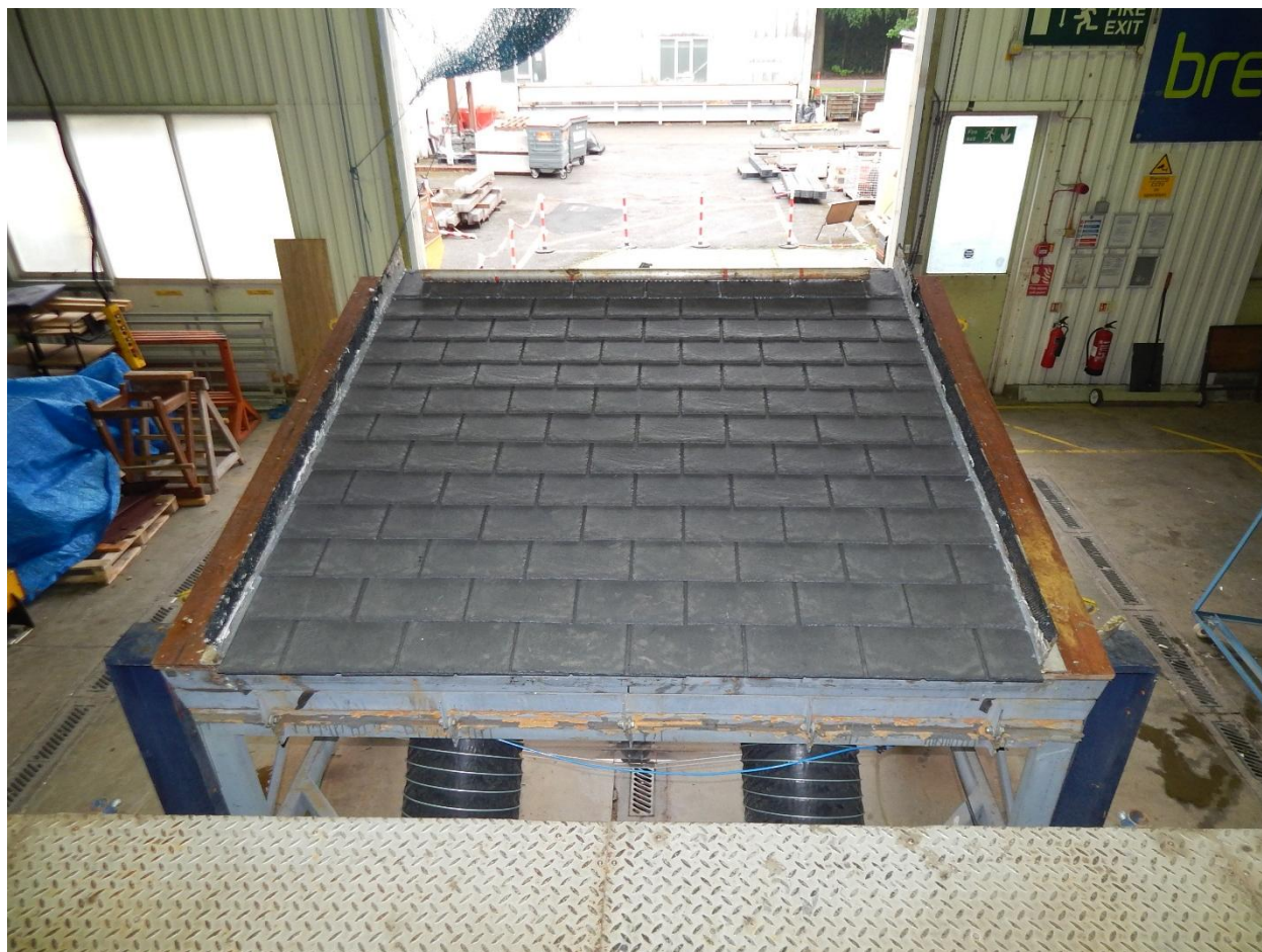
Figure 1 View of the Tapco Classic Slates installed on the BRE test rig
