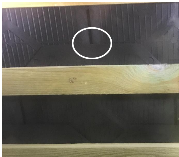
Figure 5. Image to show where leakage occurred for the Tapco Classic Slate.
