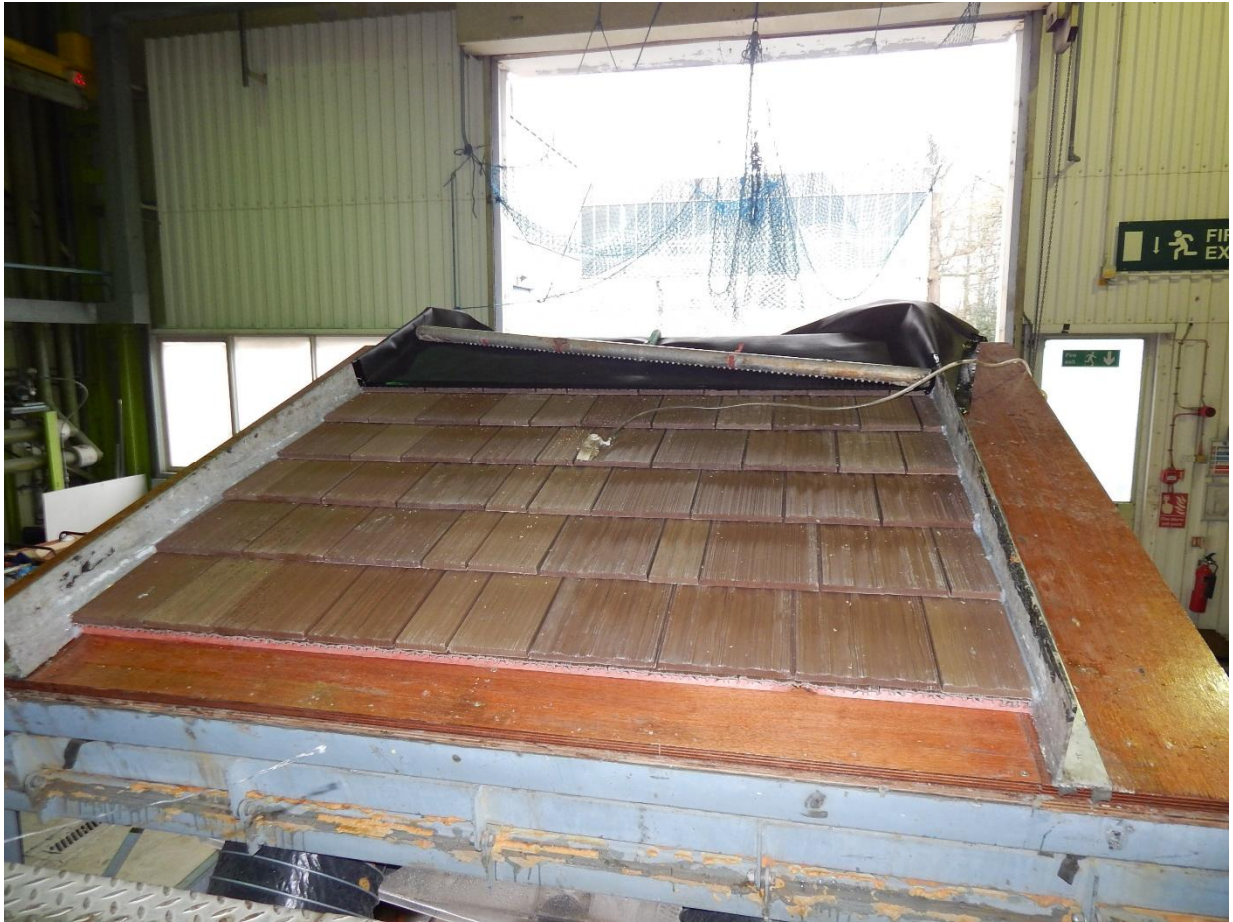
Figure 2 View of the Davinci Plastic Shakes installed on the BRE test rig.
